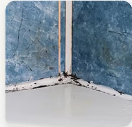
Peeling caulk or grout
