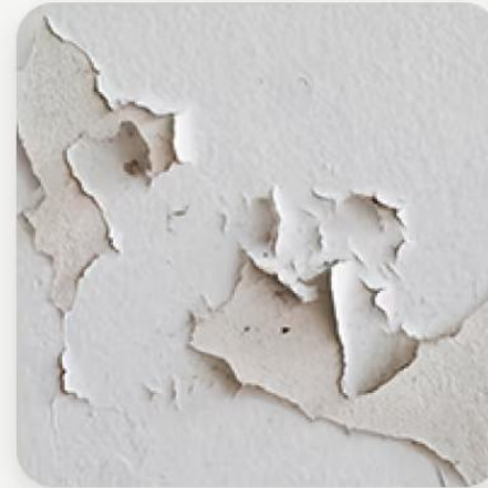
Peeling paint or wallpaper
