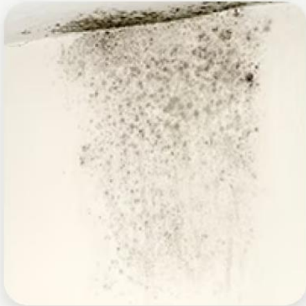
Visible mold growth
