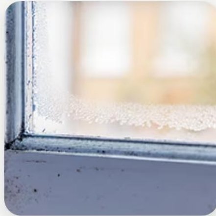
Condensation on windows or pipes
